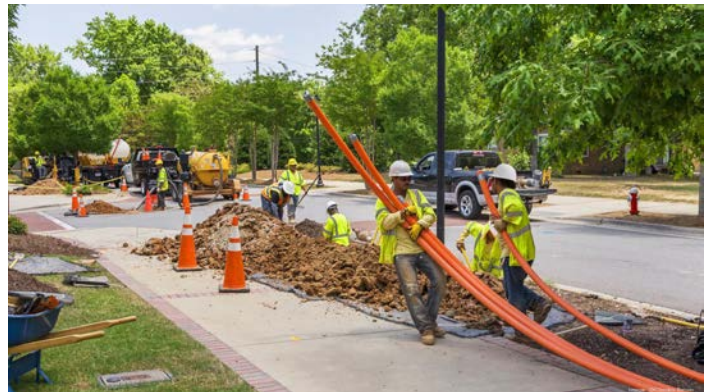
Access to fiber-optic cable networks is growing throughout Cary.
